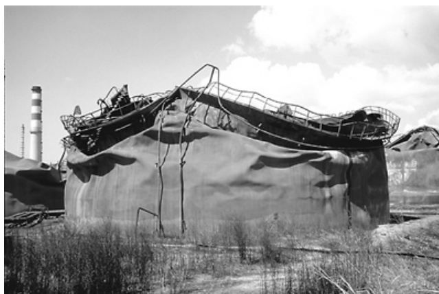
Fig. 5. Fire damage to naphtha tanks at Tüpras refinery.
