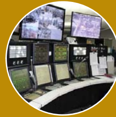
Video Cameras and Control Room
